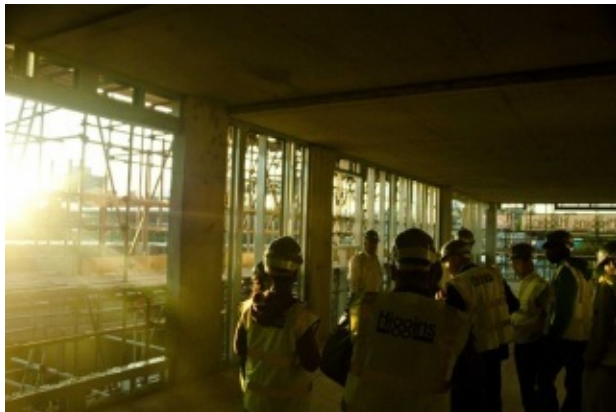
The design team and Poplar HARCA Youth Empowerment Board members on the construction site. Courtesy: Poplar HARCA
